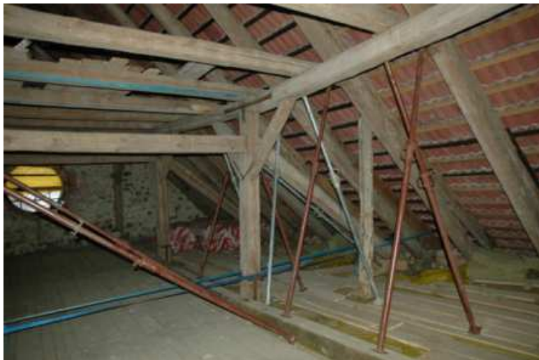
Fig. 1. Provisional bracings of wooden roof structure of historic church, endangered by building catastrophe, with a lightweight steel bracing system [2]
